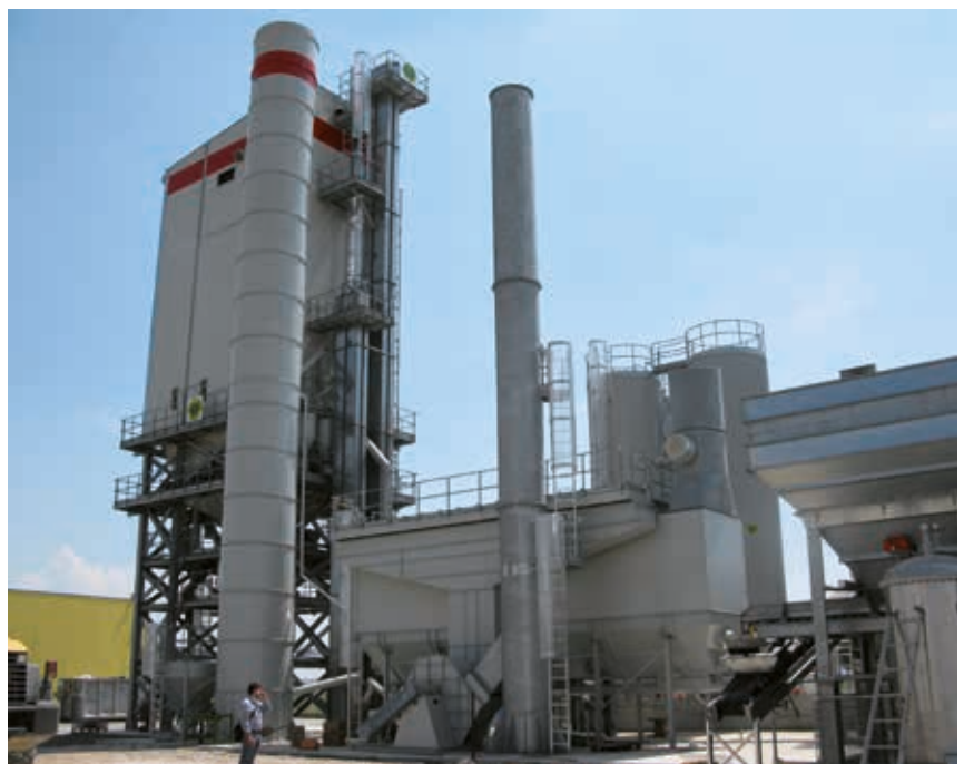
Asphalt production plant (courtesy of Bernardi Impianti)
