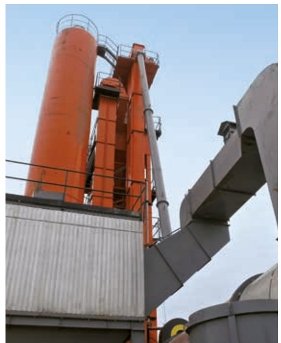
Filtering system in an asphalt production plant
