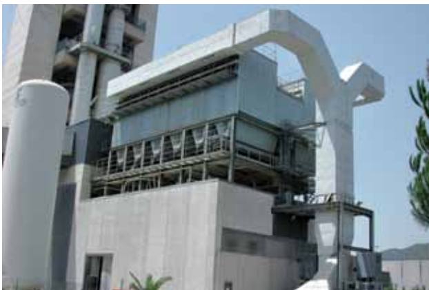
Filter in cement plant
